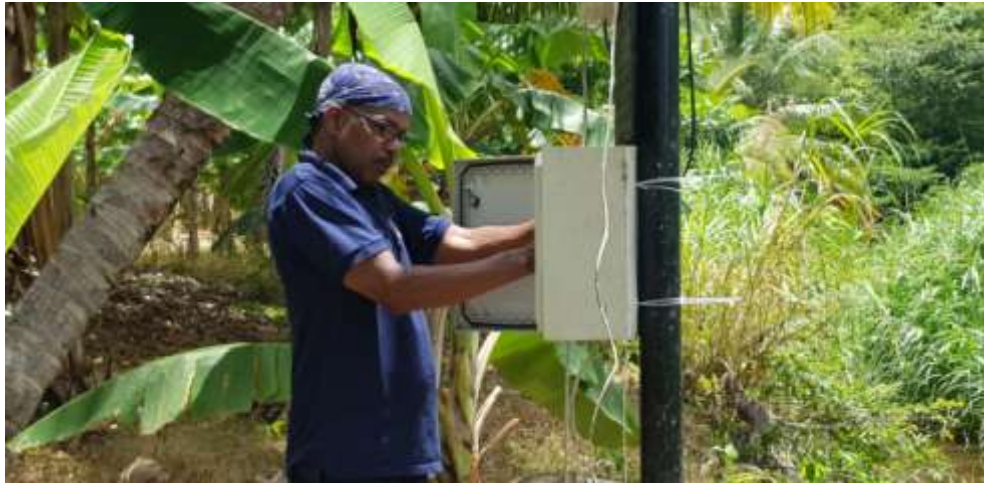
Reconfiguration of the Dennery Water Logger
