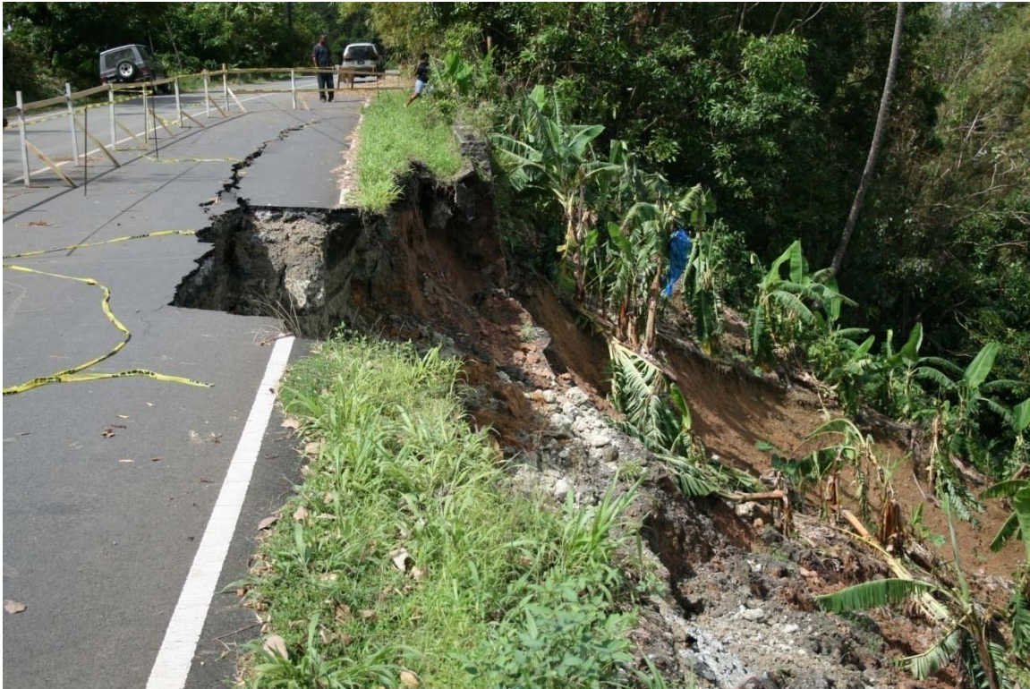
Photo 5.0 – Landslide in Barre D’Isle showing compromised roadway
