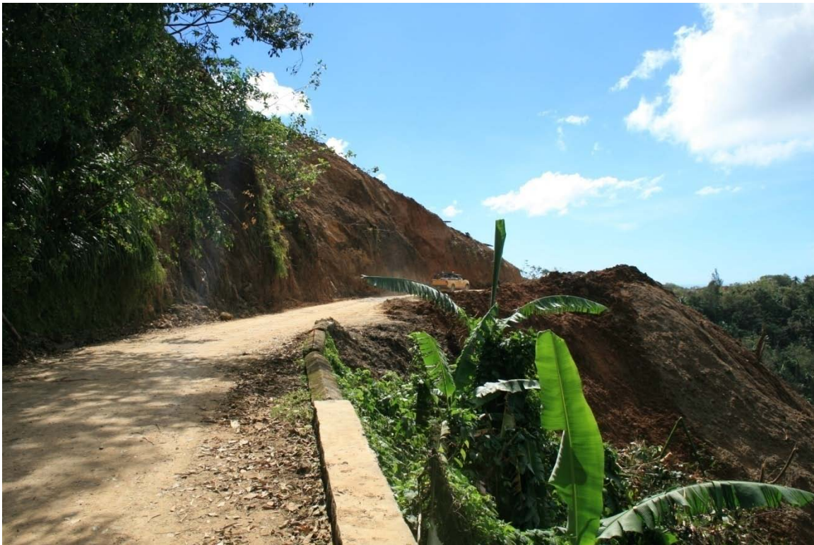
Photo 4.0 – Northern side of Colombette Landslide showing area with potential for continued debris flow
