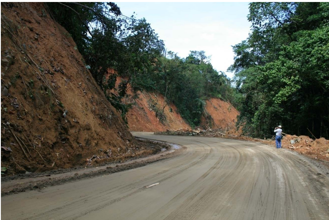
Photo 6.0 Steep slopes in Barre D’Isle Roadway which have the potential to continue sliding
