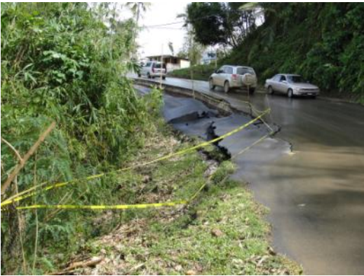
Figure 6: Road failure near LUCELEC
