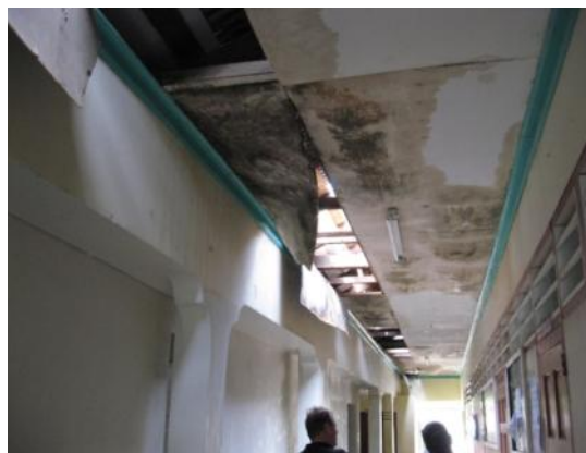
Figure 3: Evidence of roof damage at Soufriere Hospital
