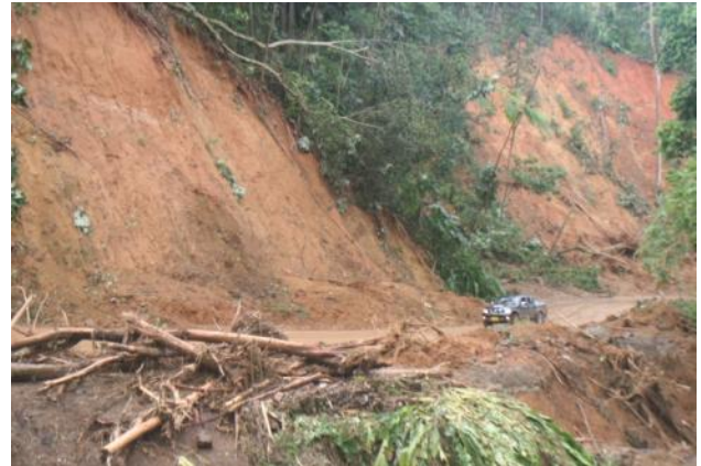
Figure 1: Landslide impacting the road infrastructure
